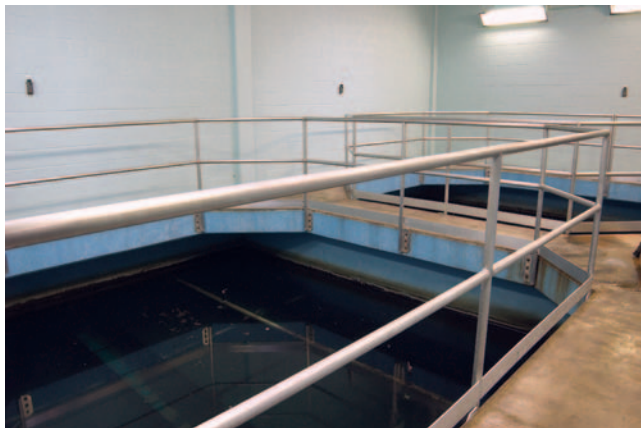
Water System Filtration Tank
